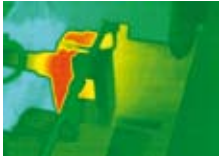
Motor: Bearing Problem
